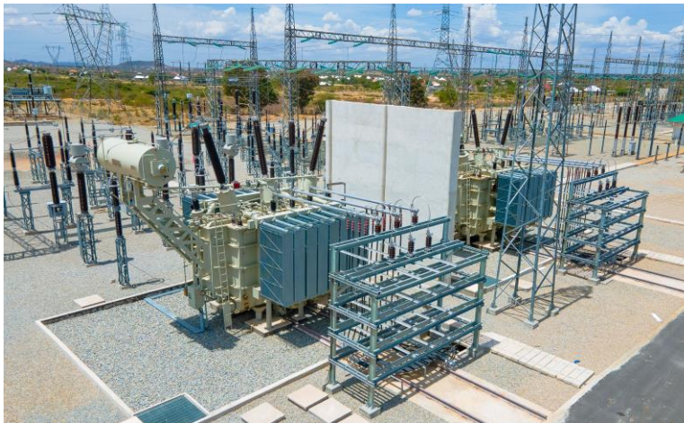
HVDC Converter Stations
