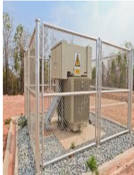
Fencing/ Protective Screen
