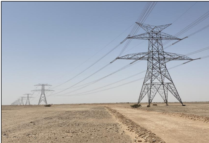
400 Kv Transmission Line, Oman
